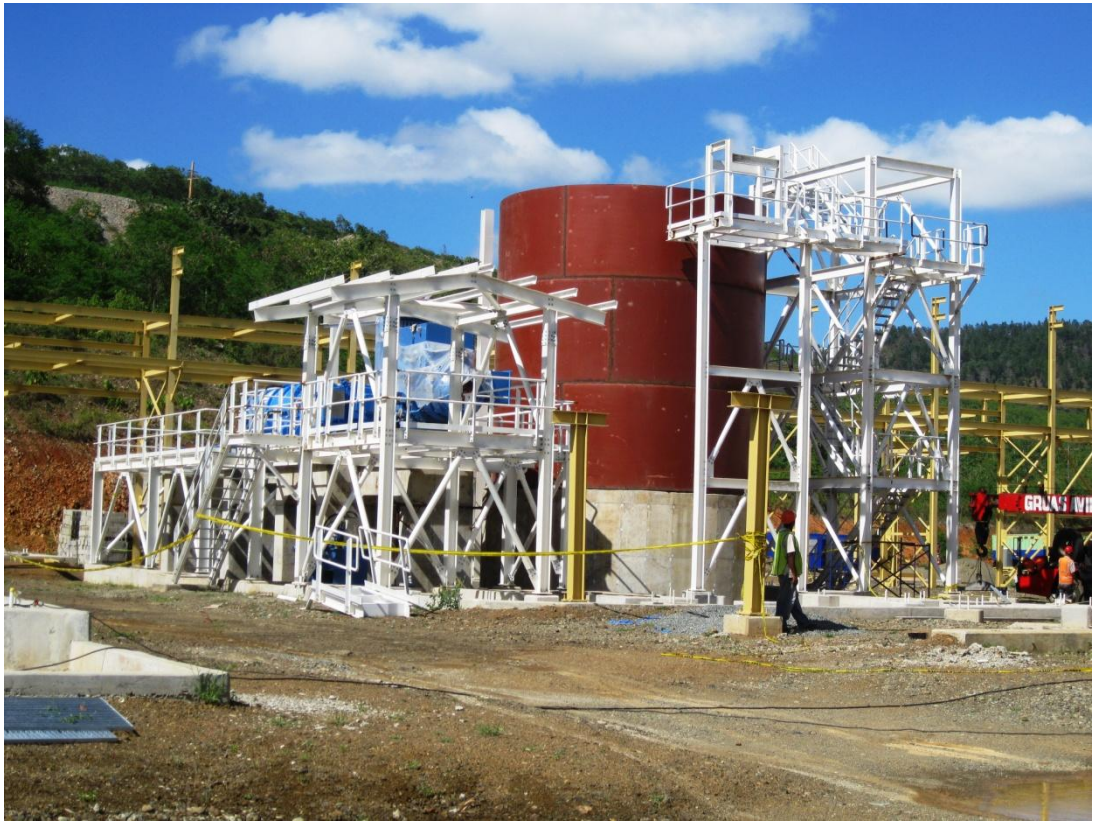
Figure 2: IsaMill & Concentrate Regrind Tank
